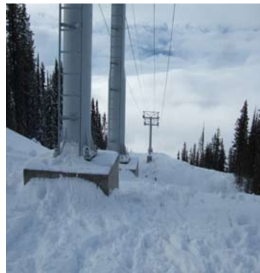
THE CABLES OF THE NEW HIGH SPEED QUAD LIFT, NAMED "THE STOKE," DISAPPEAR INTO A BANK OF CLOUDS. PHOTO: LUKE SIMPSON.
